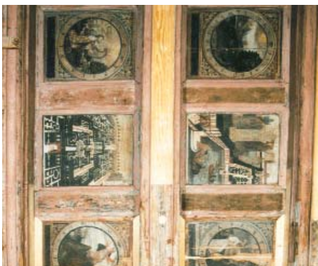
Consolidation of a damaged ceiling with nano-scaled \text{SiO}_2 at a manor's court near Riesa (source: Feinchemie Sebnitz GmbH)
